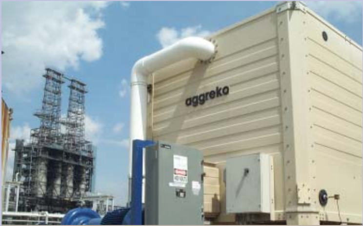
APS and Aggreko Cooling Tower Services provide innovative solutions to Lyondell-Citgo refinery.
